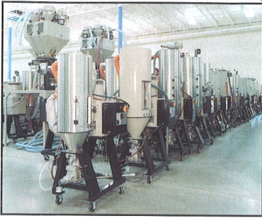
PARTIAL VIEW OF CONAIR PORTABLE DRYING HOPPERS
