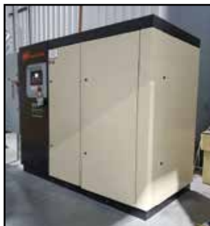
INGERSOLL-RAND 100-HP Air Compressor
