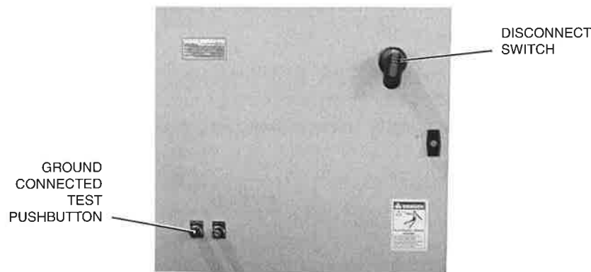
Figure 7.2-1: Main Electrical Cabinet
