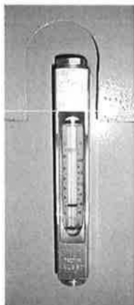
Figure 9.2-4: Hydraulic Fluid Level Gauge
